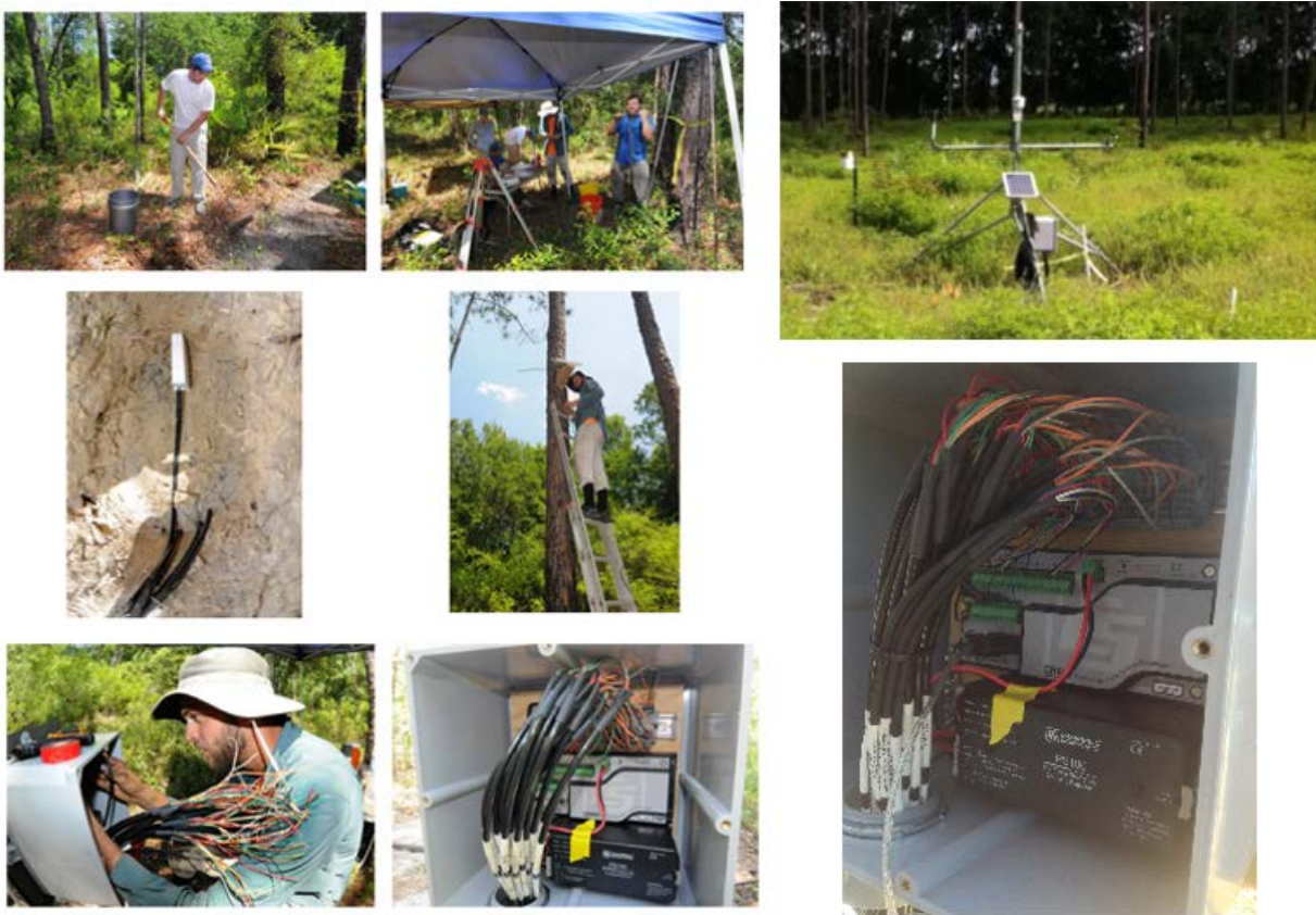
Figure 8: Photos of site installation at Little River (SRWMD). The same protocols were followed at each site, with the exception of those where the water table is deep, at which no water table recorders were installed, and additional soil moisture sensors were included. At clear cut plots in each site, we also installed a micro-meteorological station that obtains rainfall, temperature, light, wind speed, and relative humidity data.
