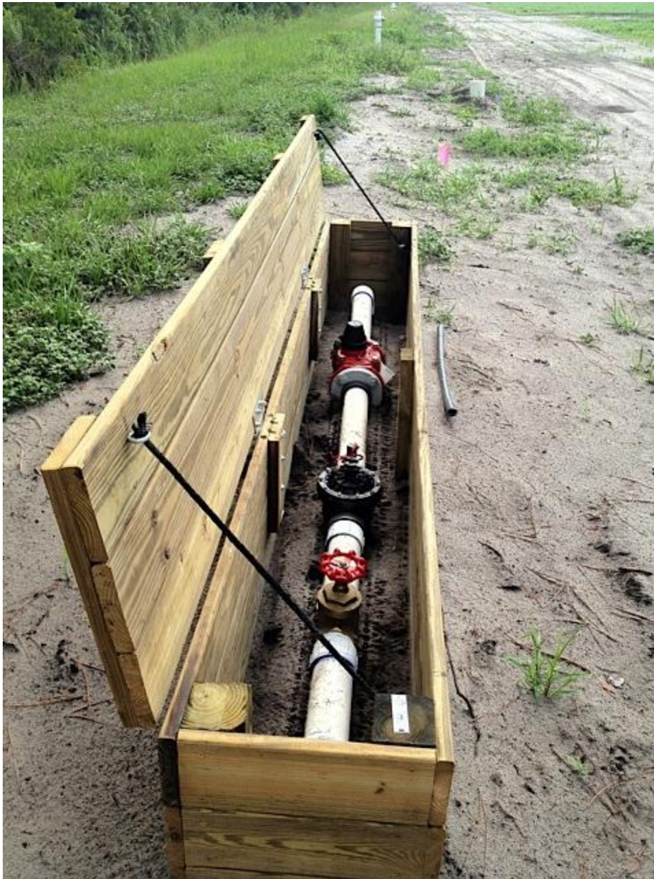
Figure 6. Sample of an irrigation system lateral for each irrigation system block/cell, complete with flow meter and solenoid valve.
