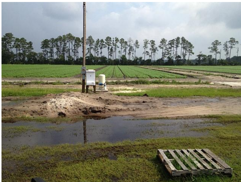
Figure 7. Well and pump station on south west corner of field.
